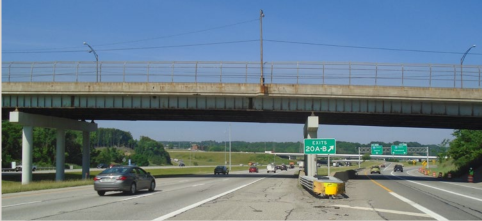
Brecksville Road Bridge prior to rehabilitation, showing deteriorated conditions
