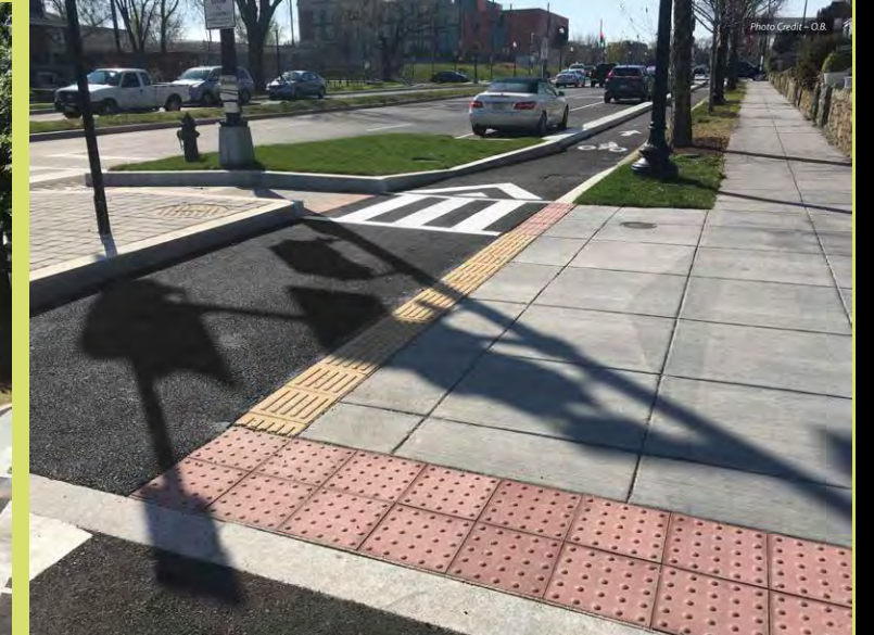
Yellow directional indicator pavers direct pedestrians toward safe crossings at the cycle track and the roadway.
