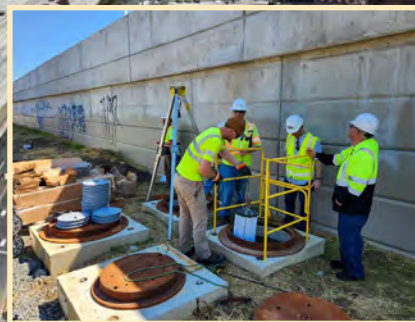
I-95's Section BS1 was the first Sector A component to use manufactured treatment devices with water quality filters.
